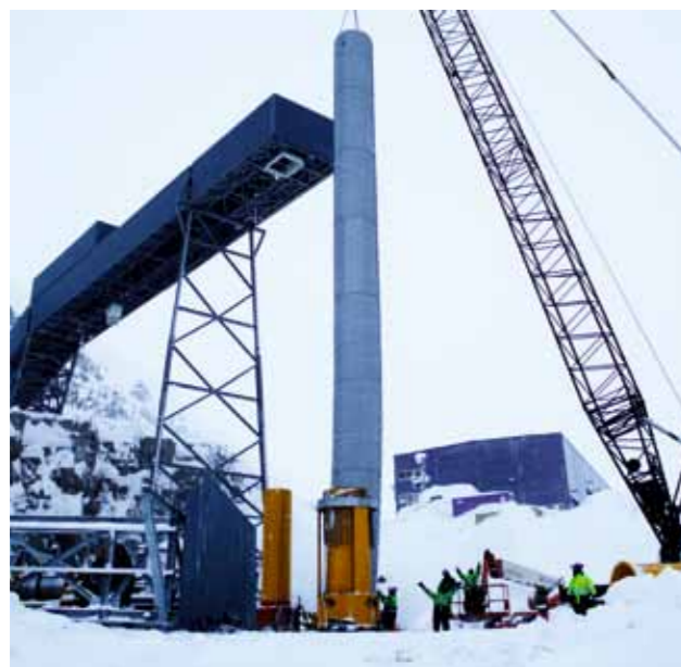
Loading of coal on stockpile (1200 t/h, -40°C, ATEX21, l=31m) during installation in Spitsbergen
